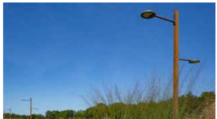
Pole lighting illuminates spaces and gathering areas that may be used late in the day (we-ef).
